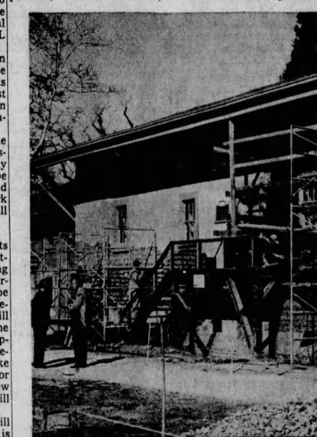
Restoration of the central building at Sutter's Fort is well under way. Workman at left behind scaffold
